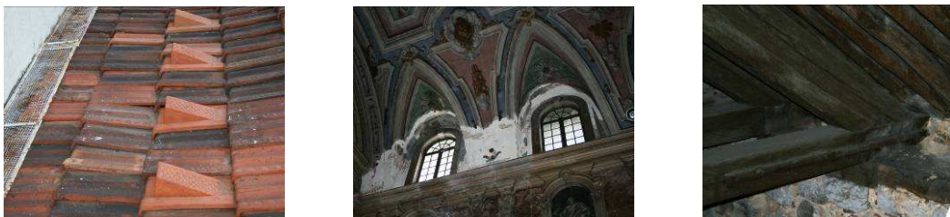
Figure 2, 3, 4 – Broken and out of joint tiles; detachment and disaggregation of interior coating; rottenness of timber elements
